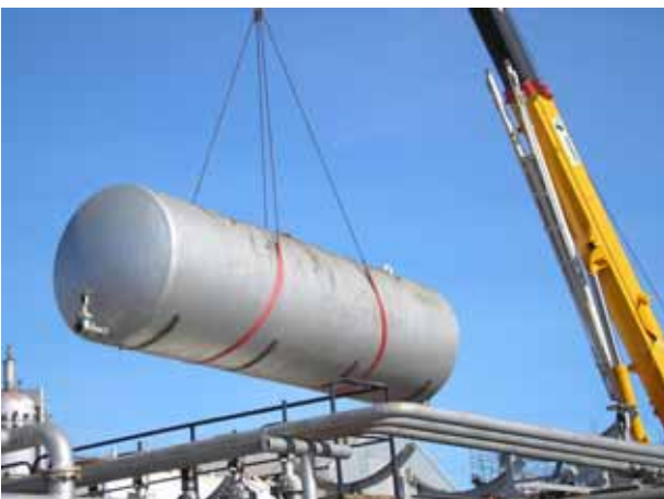
The first one hoisted out of its resting place and onto the truck ready for transfer.
