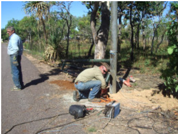
Trevor and Darren working to install the gates running off Dorat Road.
